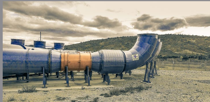
An unorthodox setup, but the best solution to this customer's short-term challenges: MC1200 in a surface installation
