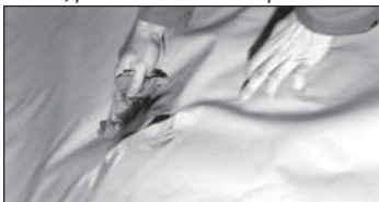
Washing of the duct textile around a tear.
